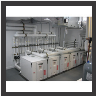
Heat Pump Systems
